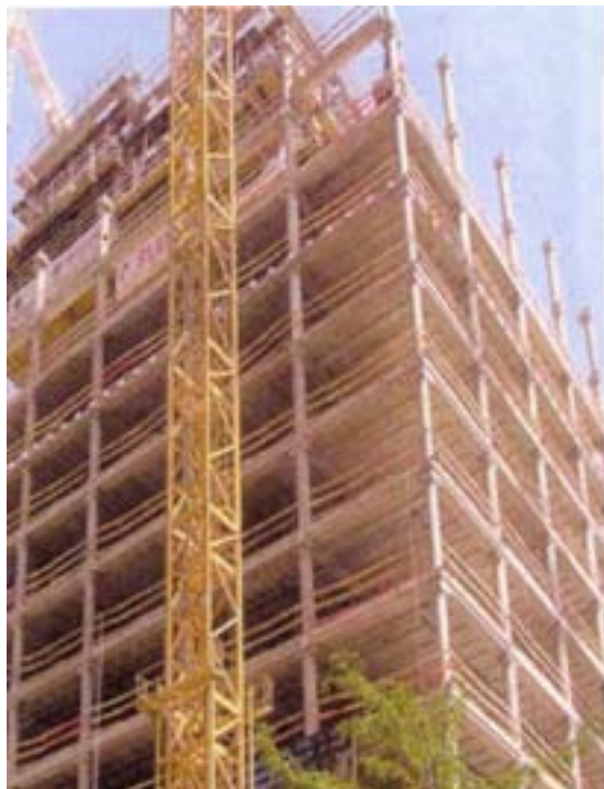
Figure 1.3: The North Galaxy Towers in Brussels. This reinforced concrete 30-storey concrete building meets the current strict requirements for fire resistance (REI 120); the columns are of high-strength C80/95 concrete. (Courtesy ERGON, Belgium)
