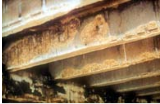
Figure CS1.2 Example of concrete elements after the fire showing spalling. (Courtesy DBV, Germany)
