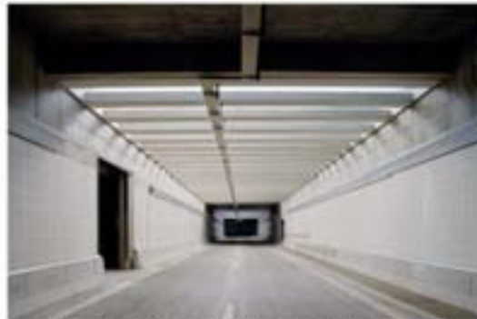
Figure CS5.2: Concrete road surfaces will stand up to the extreme temperatures encountered in tunnel fires.
